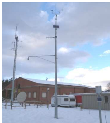
Figure 4. Exemple de station de surveillance
